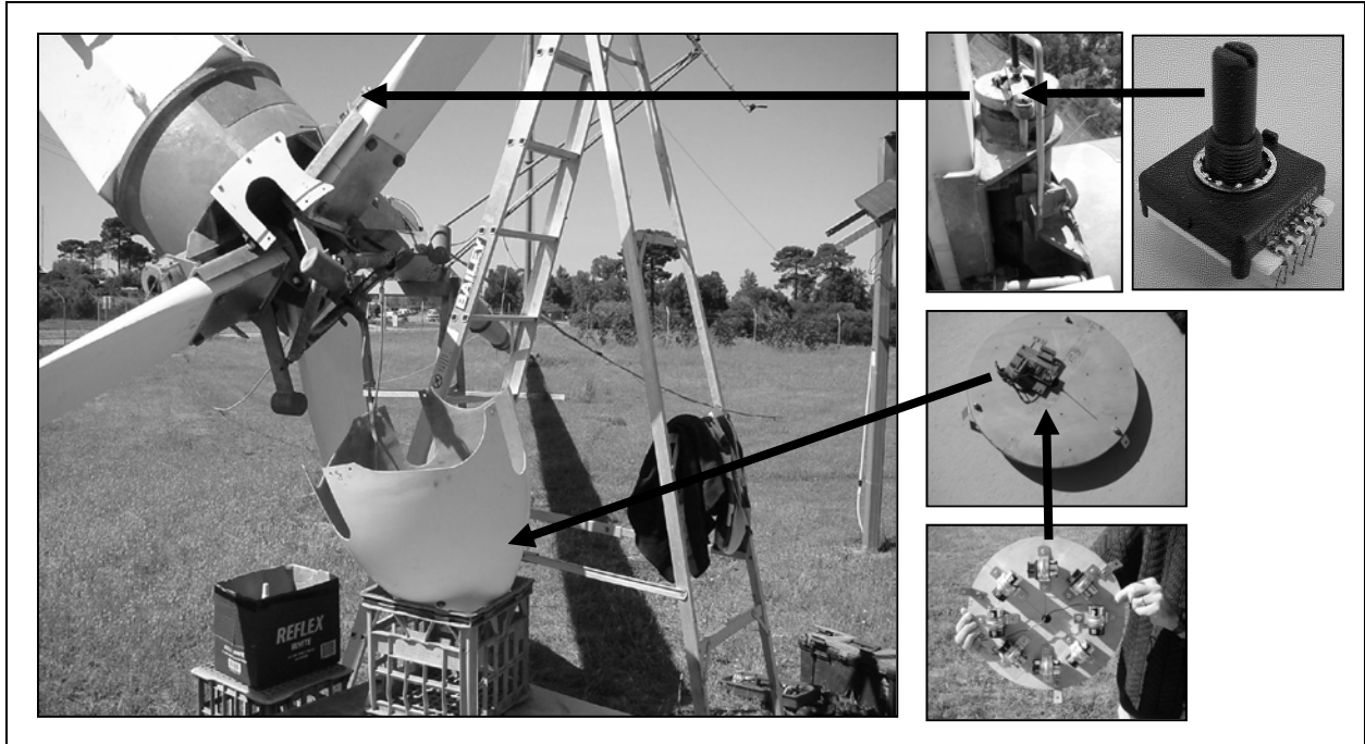
Figure 1 Installing the BPMS on a Westwind 20kW wind turbine (adapted from Stevens [13])
