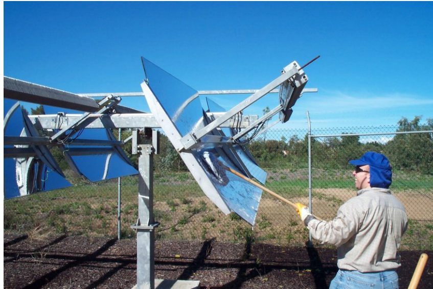
Figure 2 REE student cleaning the PV trough concentrator system at the MU Rockingham Campus
