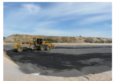
Figure 2: The drainage layer taking shape – spreading the intermediate 7mm blast furnace slag on top of the 14mm layer. Note the “air” pipes which connect to the drainage system under the slag coming up in the centre and on the batter (far end).
