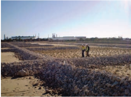
Figure 3: The initial planting stage. Note the inlet distribution pipe covered by limestone rocks and central "air" pipes sticking out.
