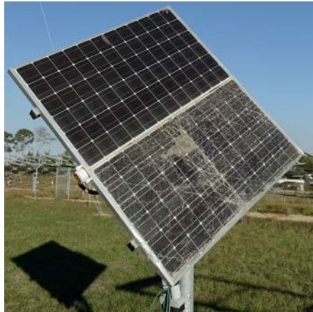
1.19 Physical impacts (fracture, glass breakage)
