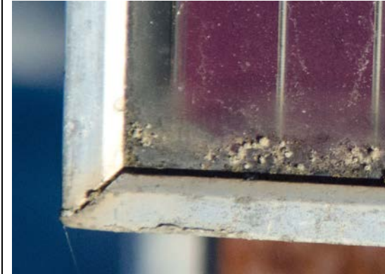
1.18 Insufficient stability of frame
