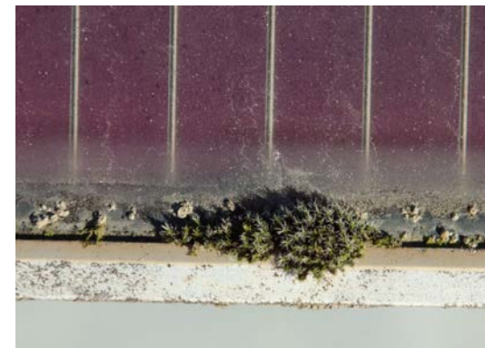
1.12 Blackening at the bottom edge of the module (ingrained dirt not possible to remove)
