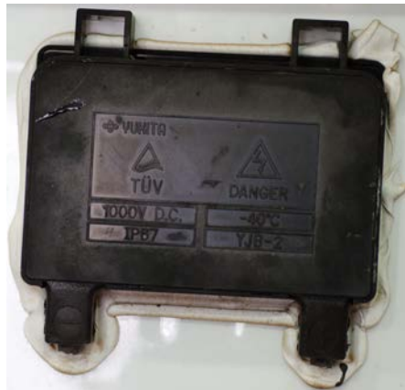
1.22 Junction box corrosion
