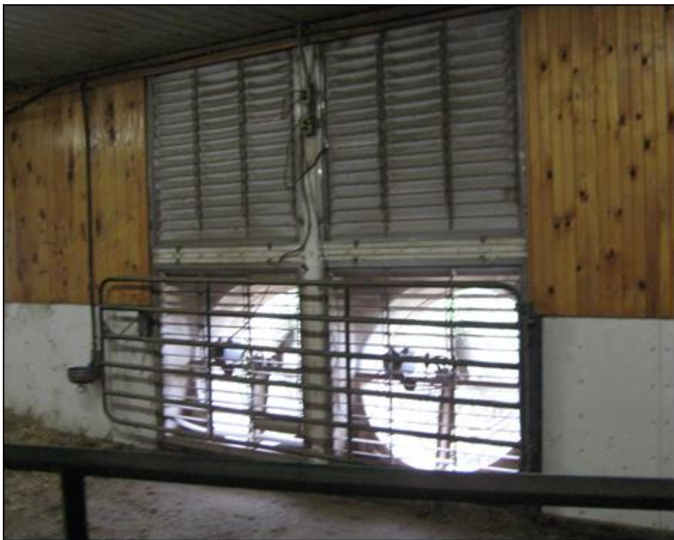
Fig. 9. Four wall-mounted fans for ventilation. Two (below) are active and two (above) are inactive at the time of taking the photograph.
