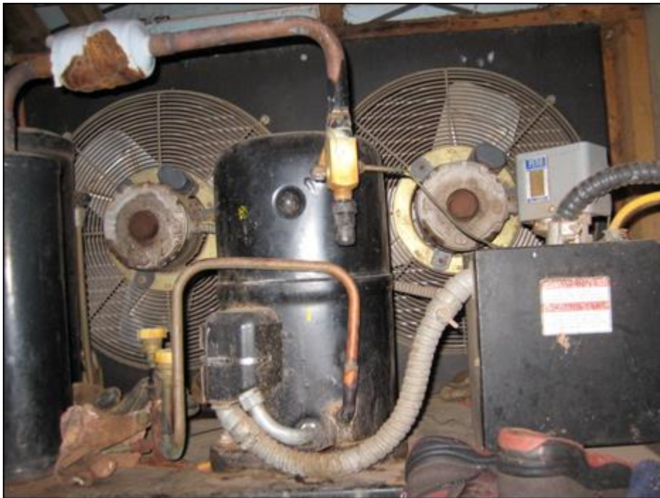
Fig. 8. One of the two 5.68 kW compressor units and corresponding cooling fans used in milk refrigeration.
