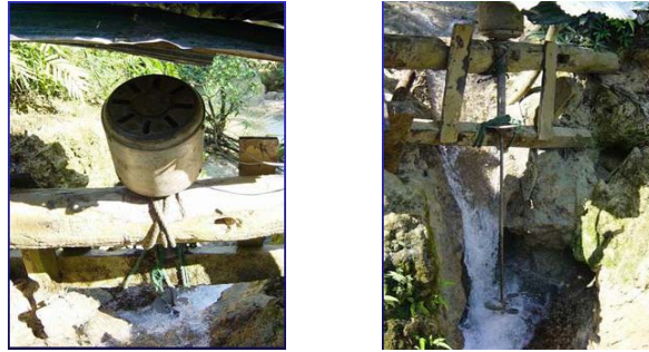
Fig. 3 The examples of pico hydro power system in Laos [1].
