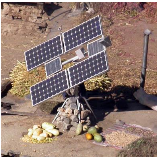
FIGURE 2: CENTRAL SOLAR PV VILLAGE TRACKING SYSTEM AT TULIN VILLAGE
