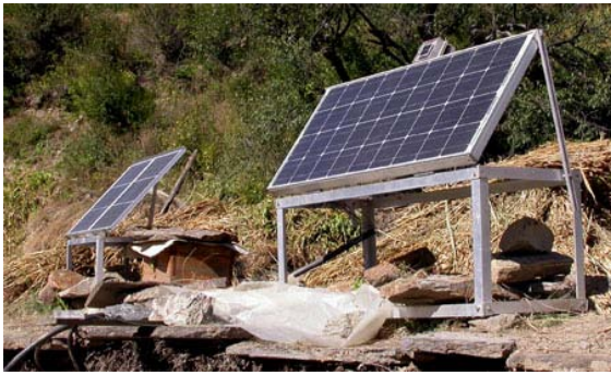
Figure 5: A solar PV cluster system for up to 12 homes. One 75W R PV module (right) generates power which is stored in the battery bank installed inside the home. All other cluster homes are connected through underground cables to the battery bank, which provides up to 3 days of power without sunshine.
